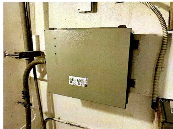
Figure 14: Main Breaker Panel
