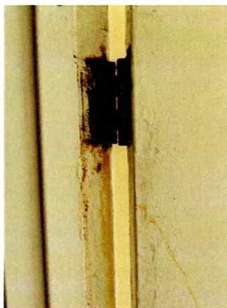
Figure 20: Signs of Corrosion at Metal Door Frame.
