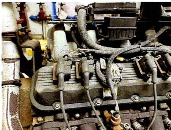
Figure 13: Condition of the Generator
