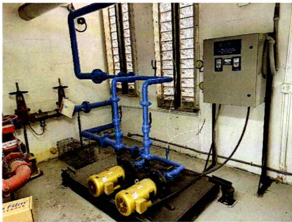
Figure 9: Existing Water Valves Installed
