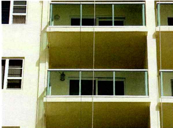
Figure 17: Actual Condition of the Balcony Guardrails
