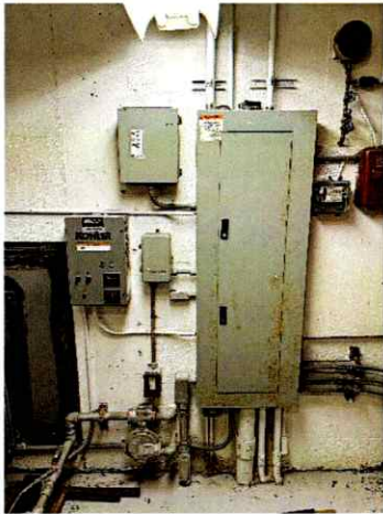
Figure 11: Main Breaker Panel
