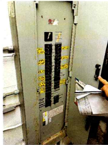
Figure 12: Main Breaker Panels
