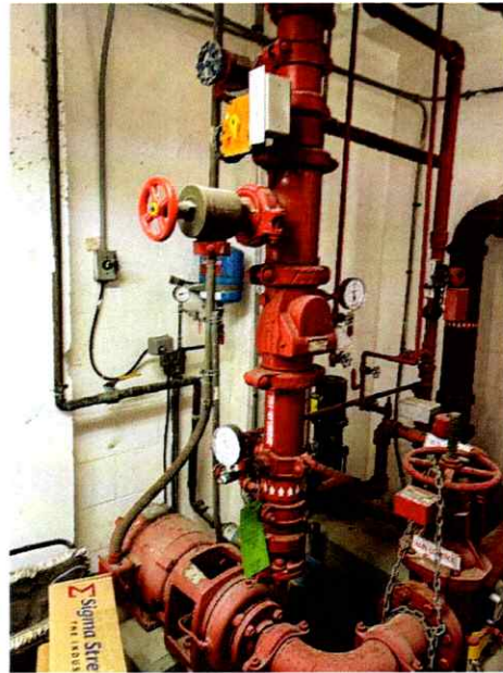
Figure 8: Fire Sprinkler System
