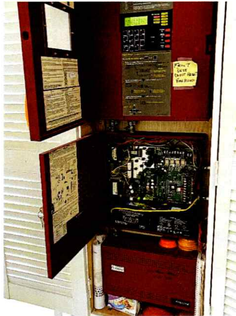
Figure 7: Fire Alarm Panel
