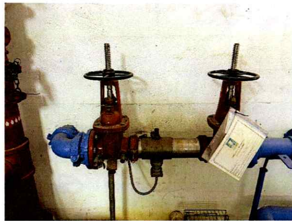
Figure 10: Main Valve of Starligh Towers
